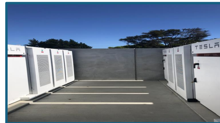
Tesla Solar Power Provision at the Vacuum Pump Station
