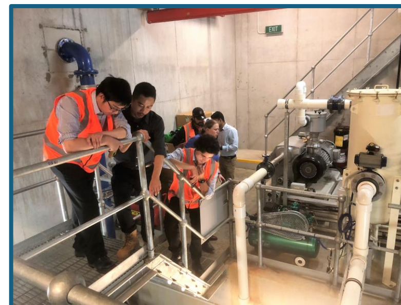
Vacuum Pump Station Training
