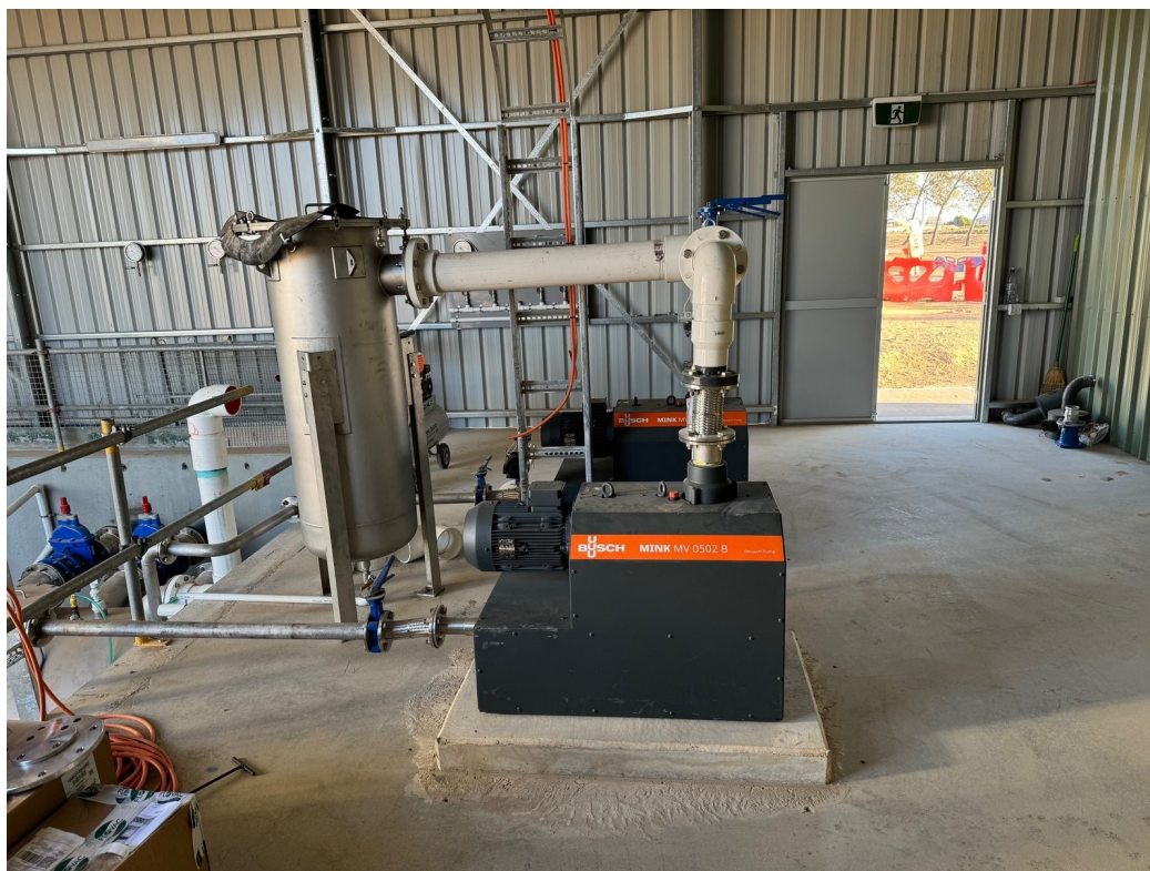
Interior of the Fishermans Bay VPS showing one of the two Bosch MINK MV 0502B vacuum pumps (foreground, label visible) and air-liquid separator (left). This pump and its standby partner, together with the two sewage pumps, represent the entire energy-consuming plant for 400 dwellings.
