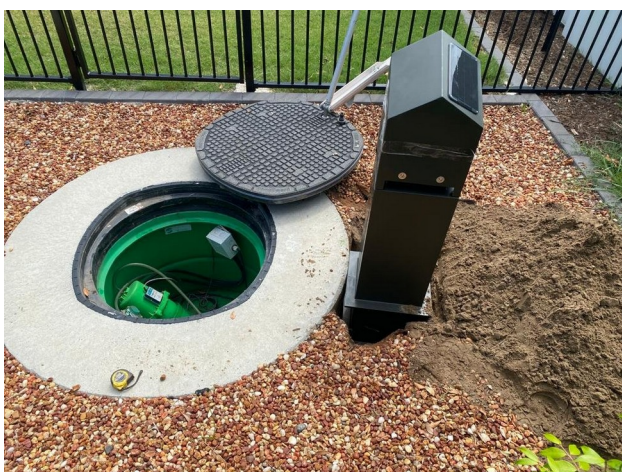
Flovac collection chamber with FV80 valve and SmartMC monitoring pillar.
