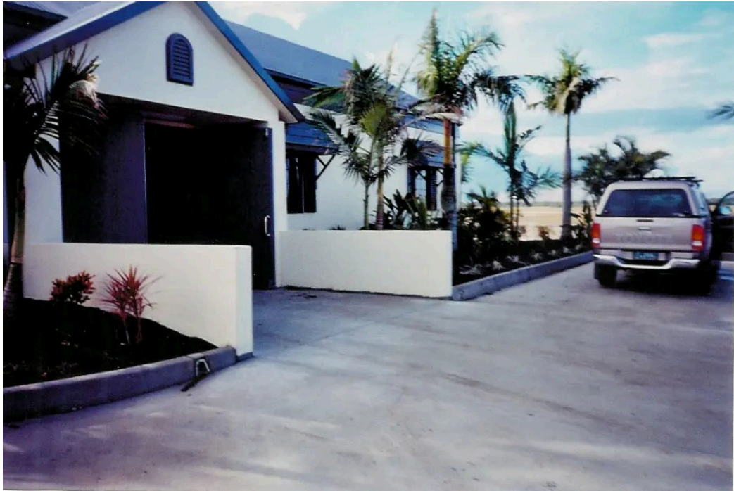
Vacuum Pump Station, this single station manages nearly 3,000 dwellings on flat land and is the only place where electricity is required.
