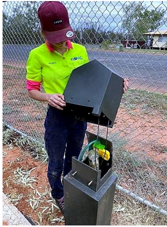
A Flovac operator at a monitoring pillar with a remote mounted controller
